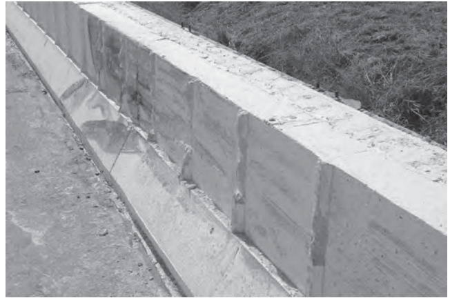
Figure 68. Barrier damage for Crash Test 1.
