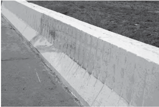
Figure 70. Barrier damage for Crash Test 2.
