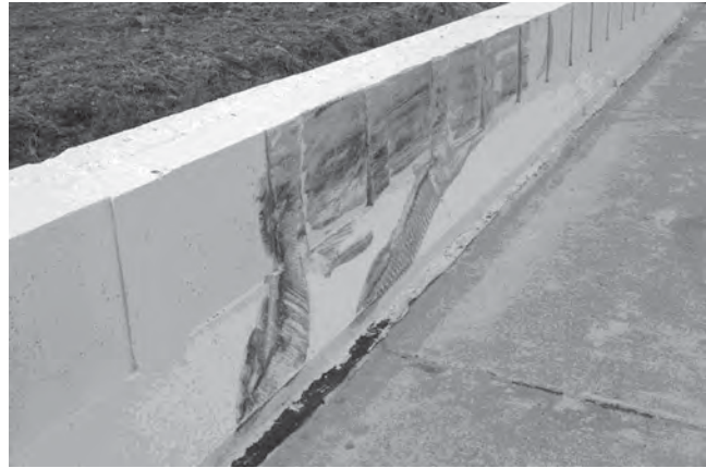
Figure 76. Barrier damage for Crash Test 5.
