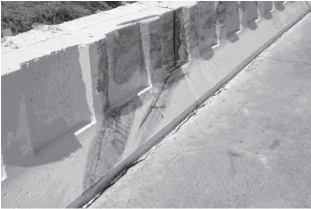
Figure 81. Barrier damage for Crash Test 7.
